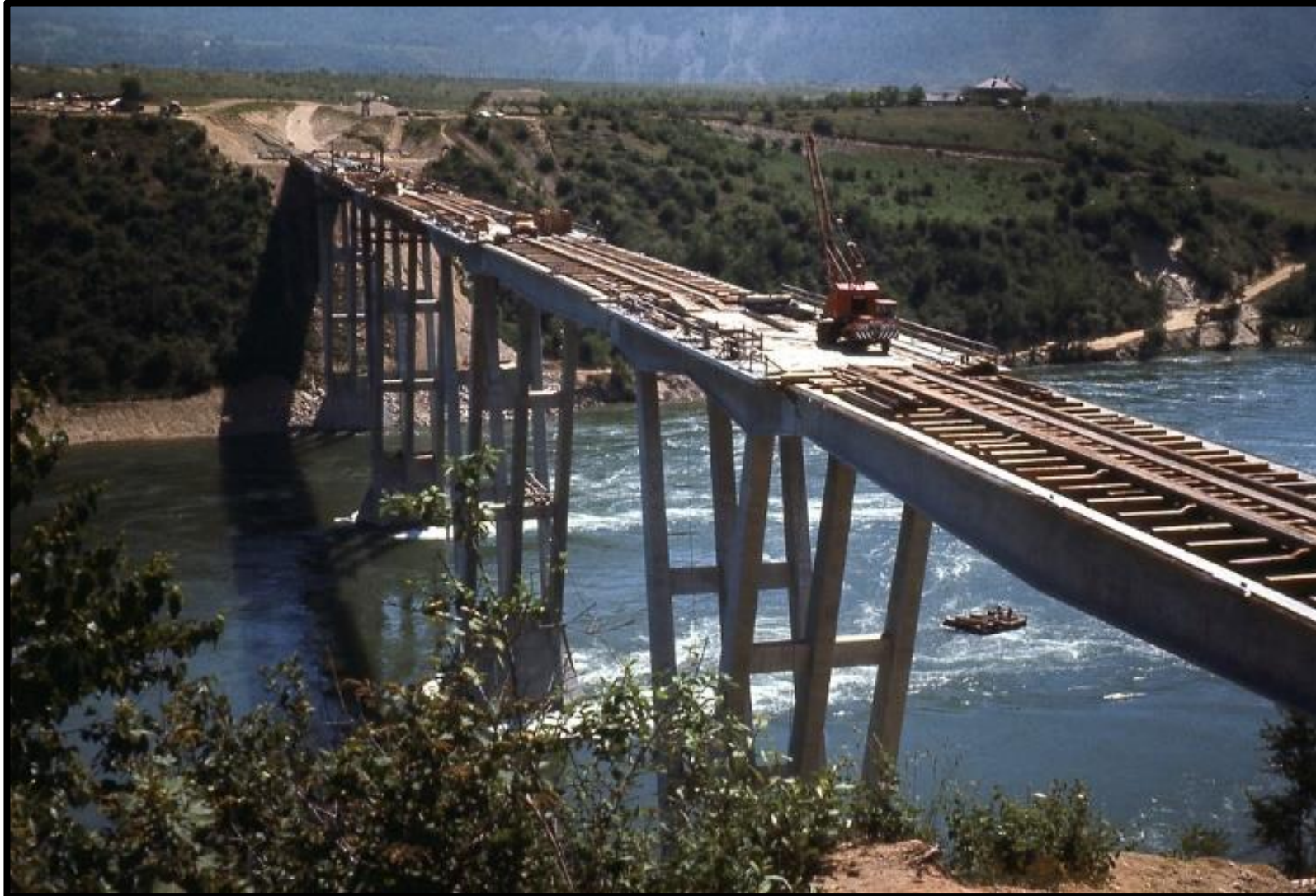
24. Columbia River Bridge at Castlegar. Constant engineering of new roads and bridges.
